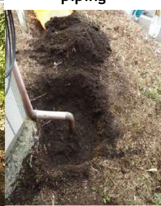
removing a "hot spot" at the bottom a discharge pipe of a gutter
