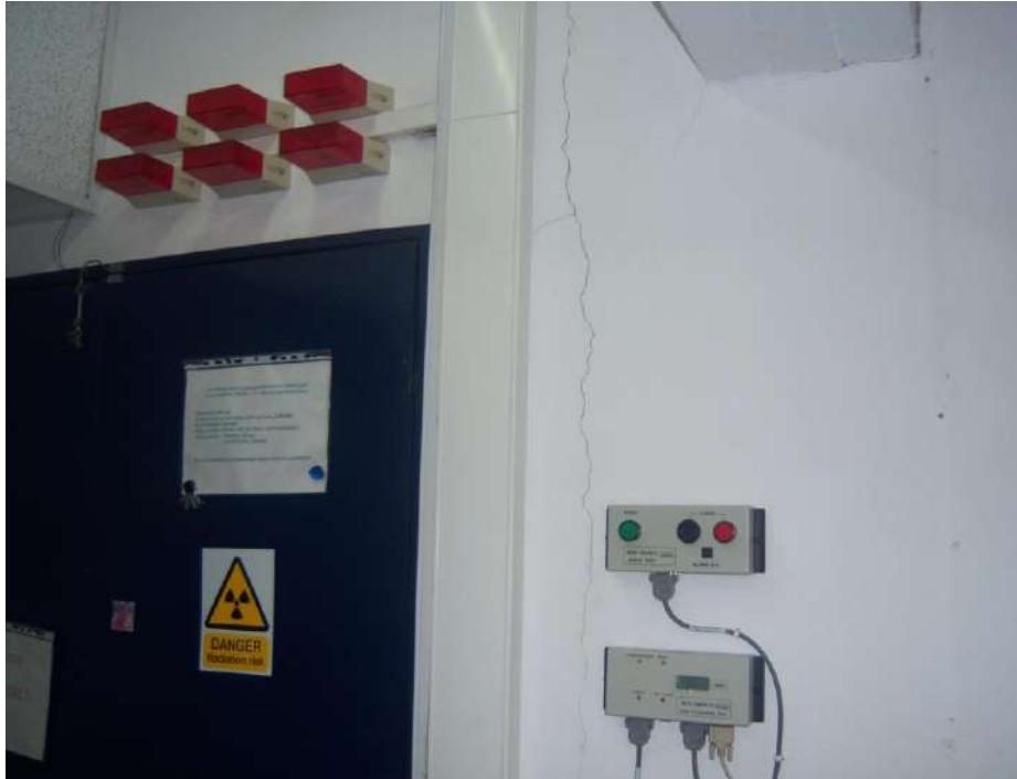
Flashing lamps and alarm monitor
